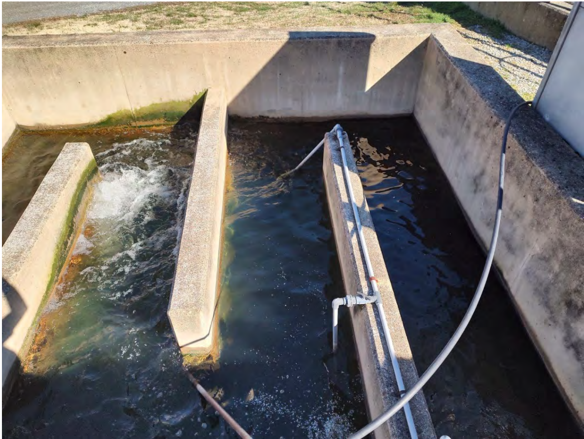
Figure 5.2.4 Chlorine Contact Basin
